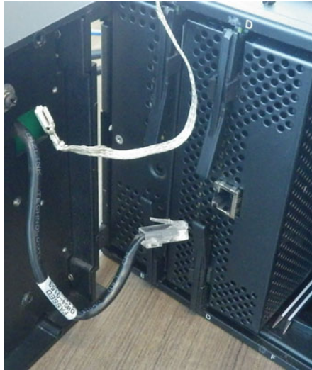
Figure 11-16: Disconnected ground cable and CPU connector
